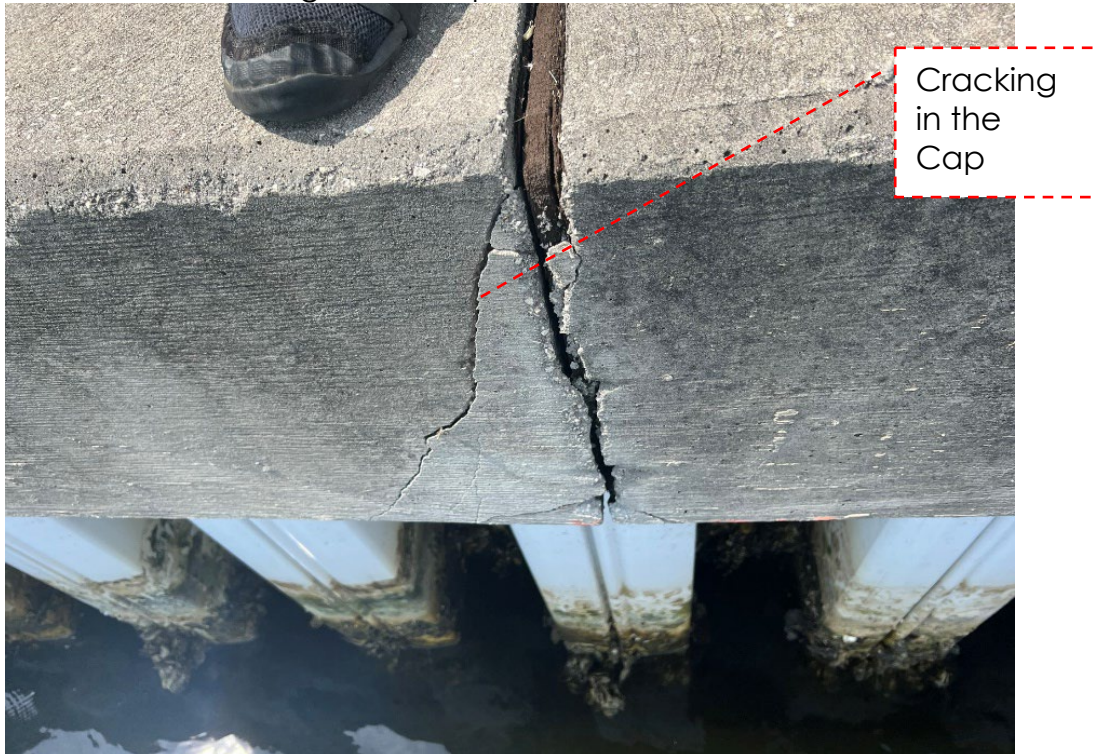
Photo #3 – Cracking in the Cap.
