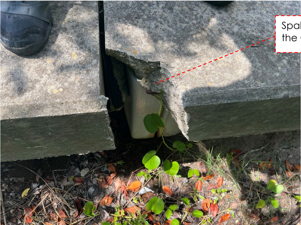
Photo #7 – Typical Spalling of Concrete Cap.
