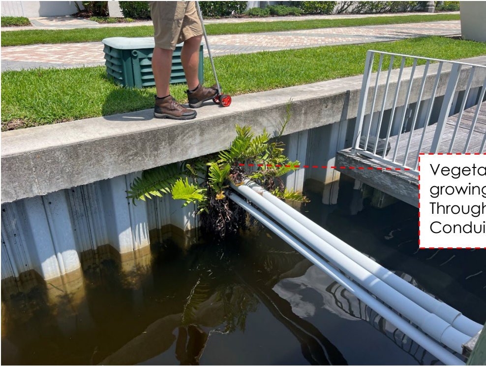
Photo #5 – Vegetation growing Through Conduit.
